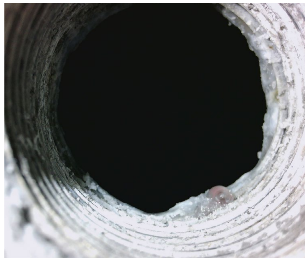
Aluminum hydroxide corrosion
